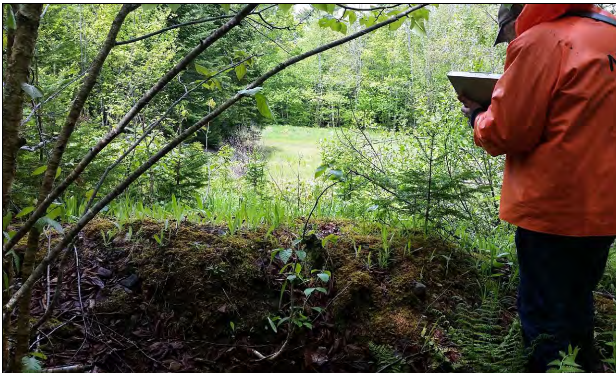
Figure 20. Berm at the bottom of slope, north of the quarry. An unnamed access/logging road is visible in background (June 10, 2016).
